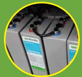
Deep-cycle long life, mainteance free batteries
